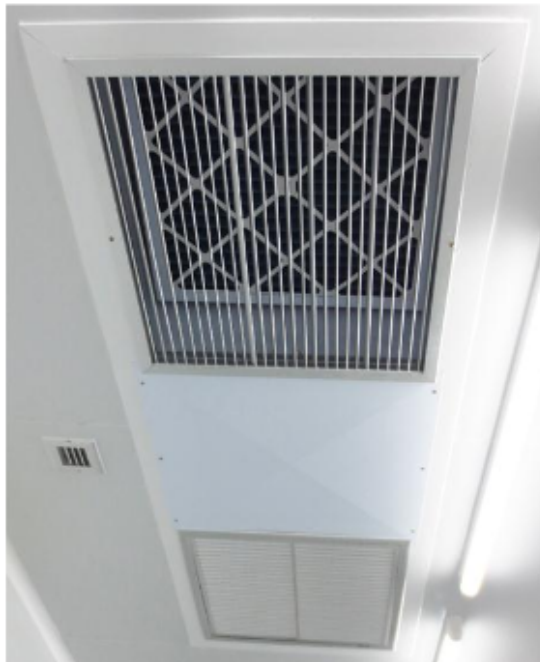
Cleanroom Air Filtration Unit (CRCM)
